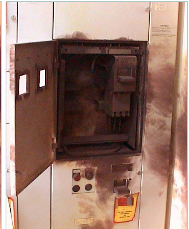
Figure 1-5. Inside of MCC bucket after breaker was removed
