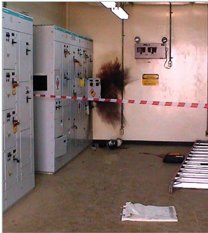
Figure 1-3. Utility room post-event
