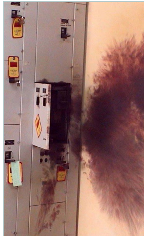
Figure 1-4. Burn on wall adjacent to MCC
