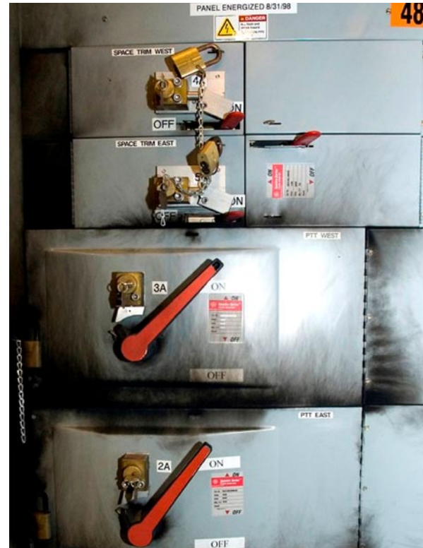
Figure 1-1. Electrical panel PB-1 with switch 3A in the center with signs of arc flash (soot)
