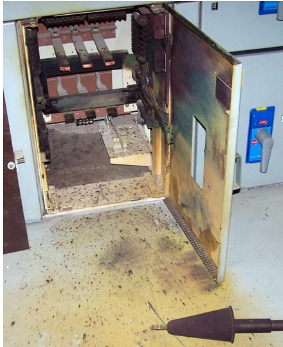
Figure 1-3. The damaged spare 480-volt circuit breaker cubicle and hot stick on scorched floor
